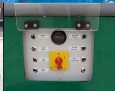
Covered Control Panel
